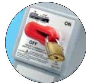
Handle with padlock installed
